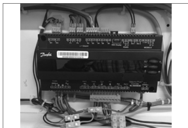
Picture 5 : Temporary wiring
