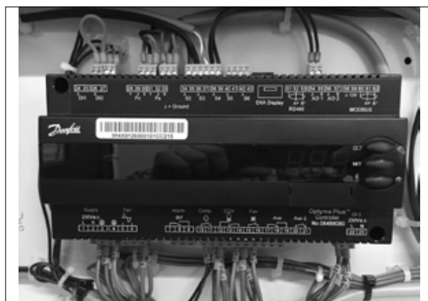
Picture 4 : Normal wiring
